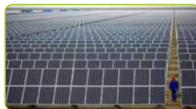
solar electric field in Gansu
